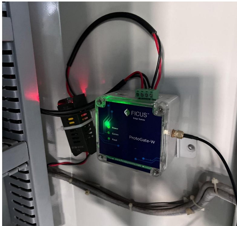
Image 3: Above image shows the Ficus Device Installed on the Chiller Panel
